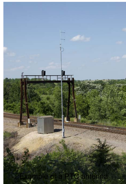
An example of a PTC antenna structure near other railroad signals.
