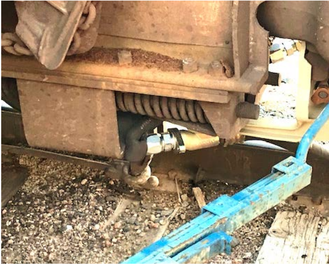
Figure 2. Kinked intermediate end-of-railcar air hose that was discovered during an inspection after an end-of-railcar air hose configuration was incorrectly applied. (Photograph provided by UP.)
