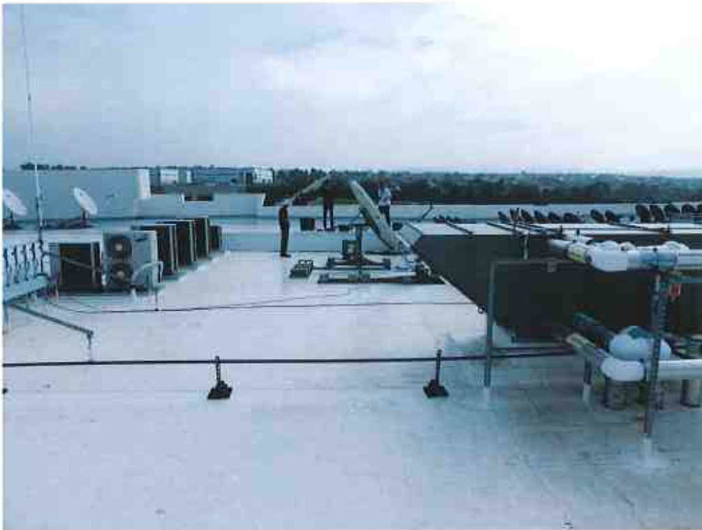
View of transmit antenna looking south
