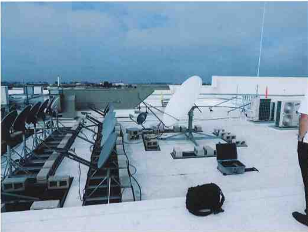
View of transmit antenna looking west
