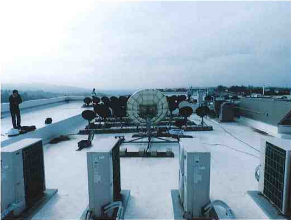
View of transmit antenna looking south
