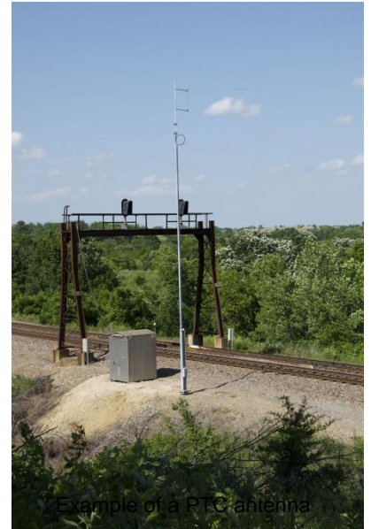
An example of a PTC antenna structure near other railroad signals.
