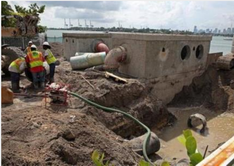
Stormwater pump – Miami Beach, FL
