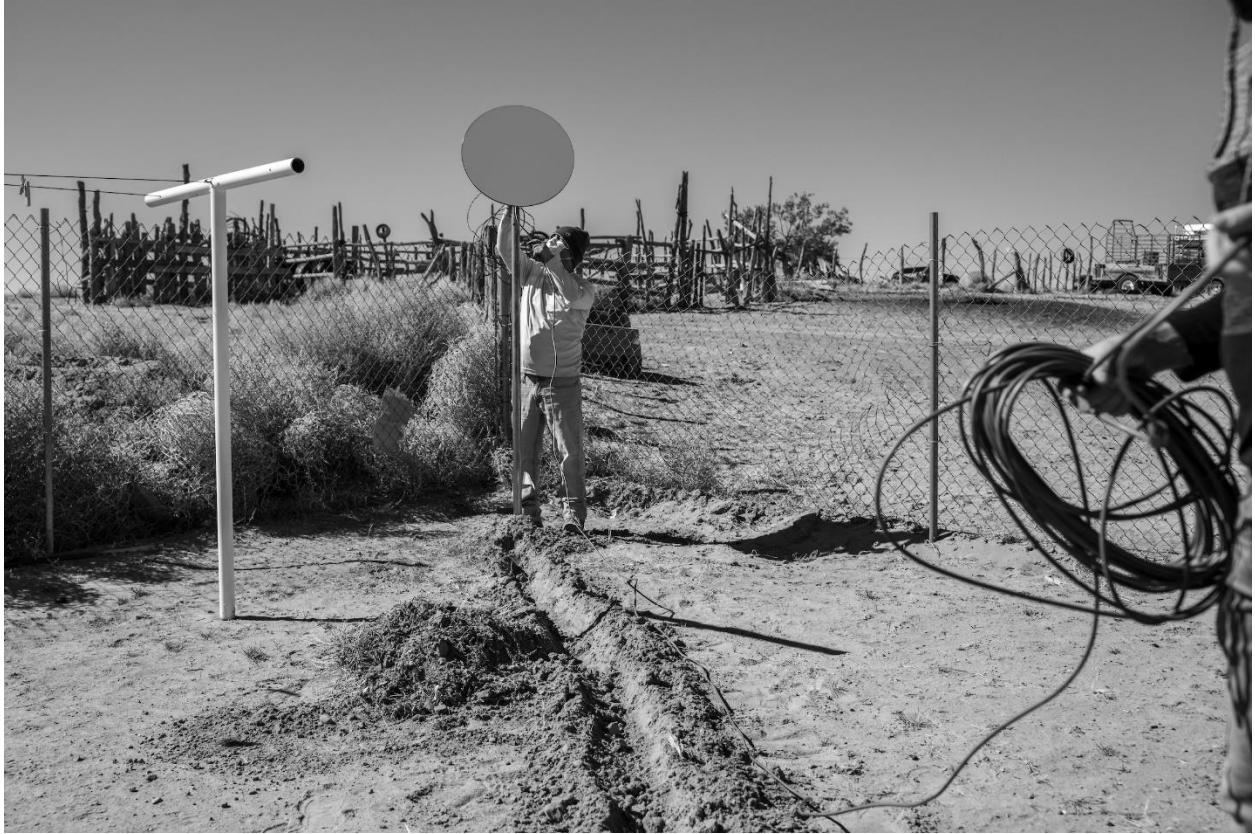
Setting up Starlink on a pole, away from livestock
